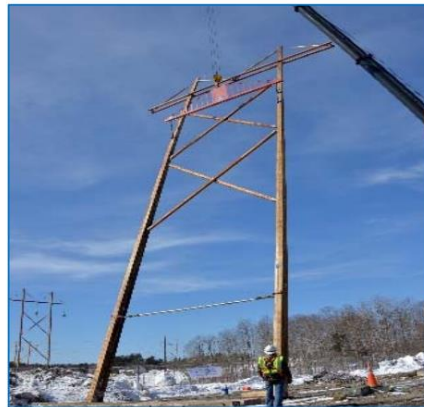
Modernizing existing assets
